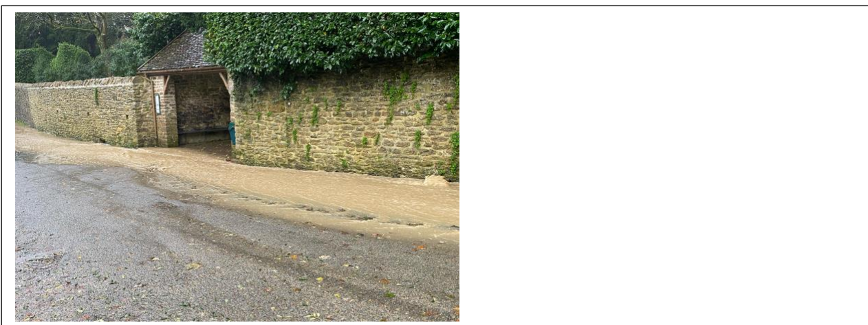
Figure 7 On 31 October 2021 nearly 4 inches of rain fell in two hours causing surface water flooding in the villages of Puncknowle, Swyre and West Bexington.
